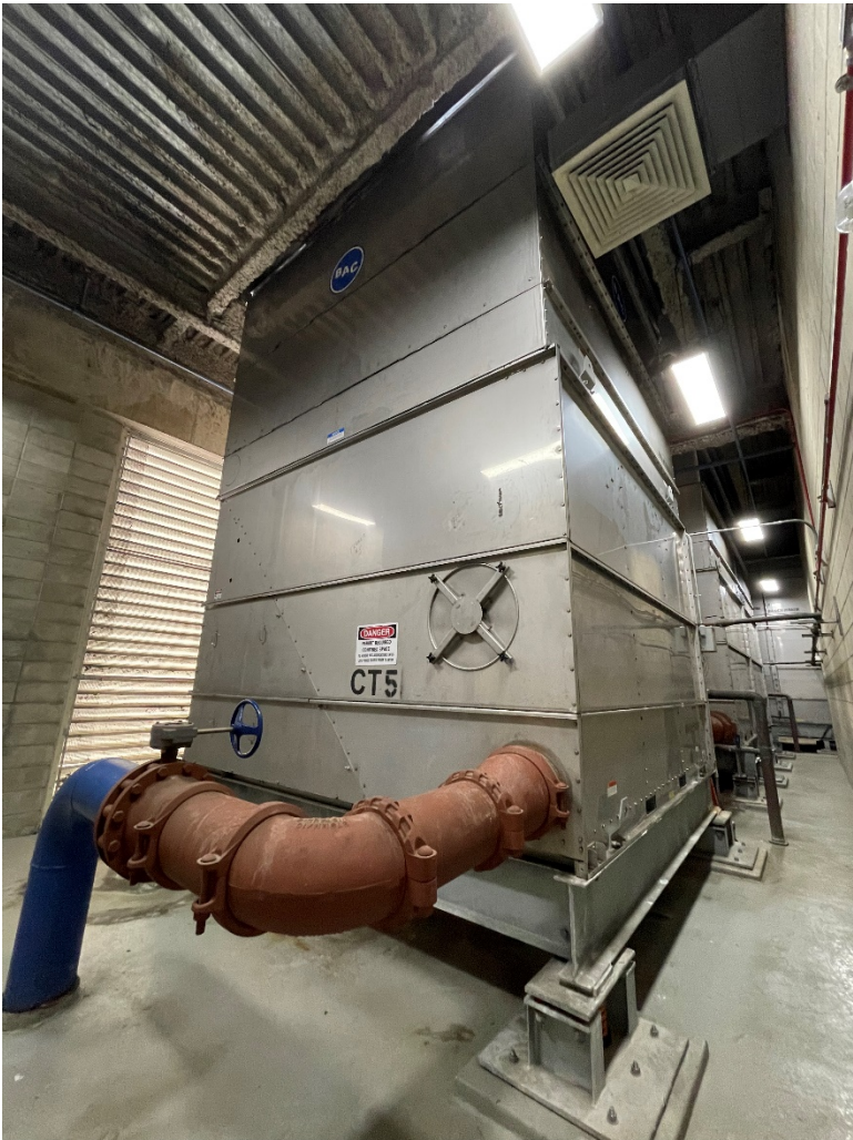
Cooling Tower #5 Lower Section (BAC VT1-400-Q #U164431106-01-01)
