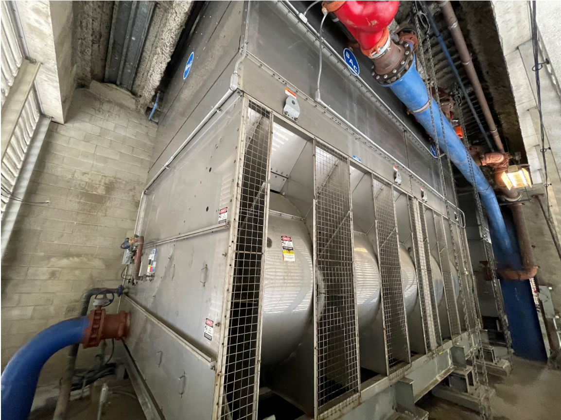
Cooling Tower #1 Lower Section (BAC VT1-800-Q #U164431105-04-01)
