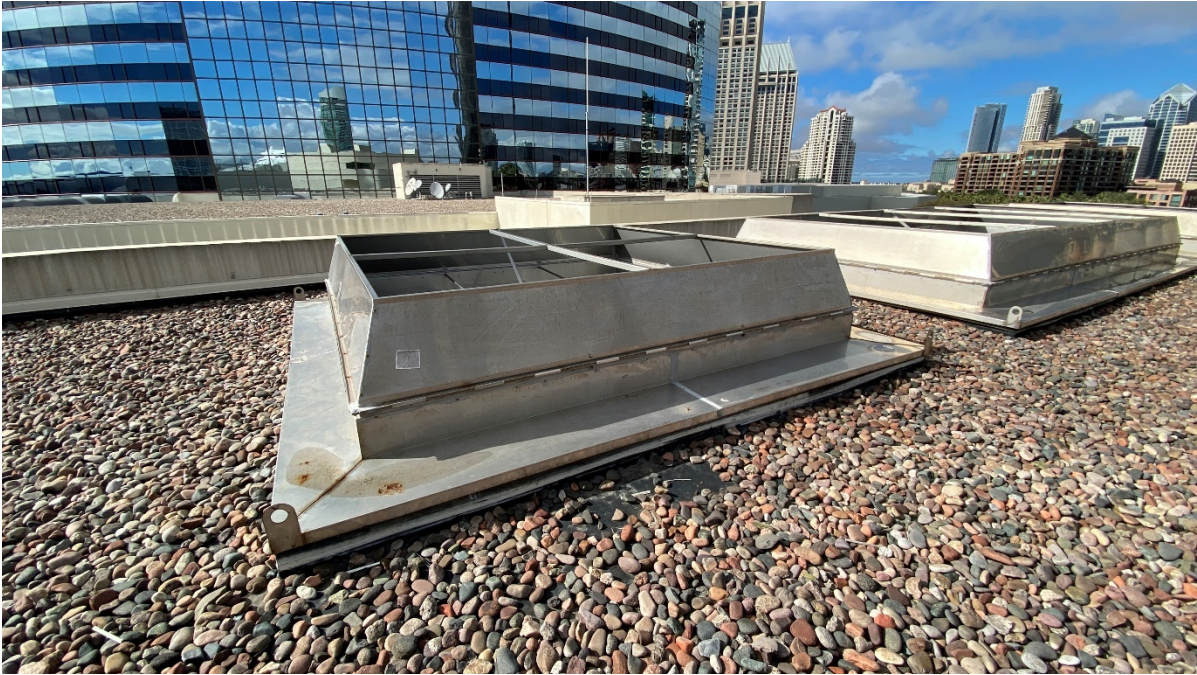
Cooling Tower #5 Top (BAC VT1-400-Q #U164431106-01-01)
