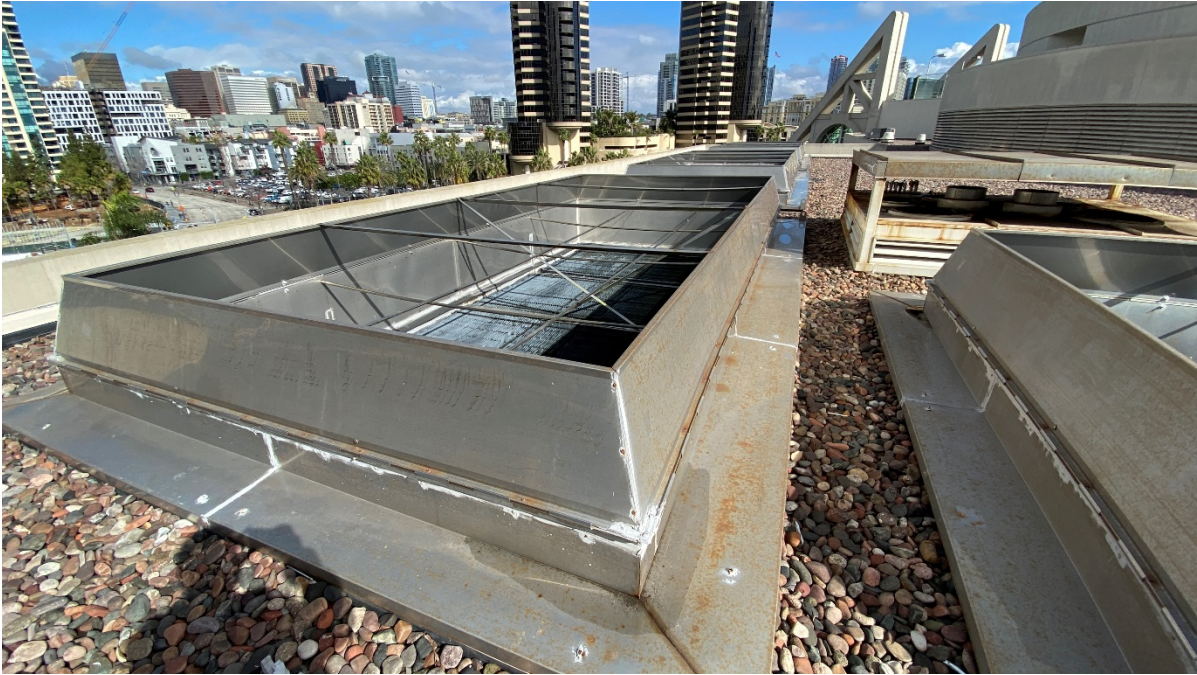
Cooling Tower #3 Upper Section (BAC VT1-800-Q #U164431105-02-01)
