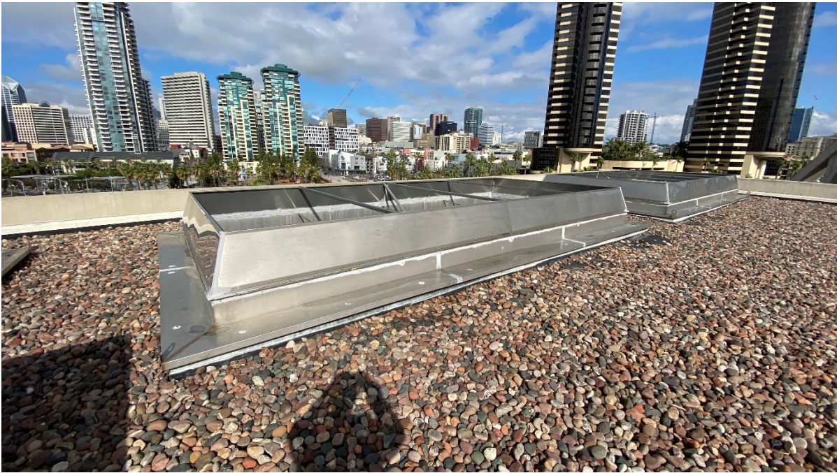
Cooling Tower #2 Top (BAC VT1-800-Q #U164431105-03-01)
