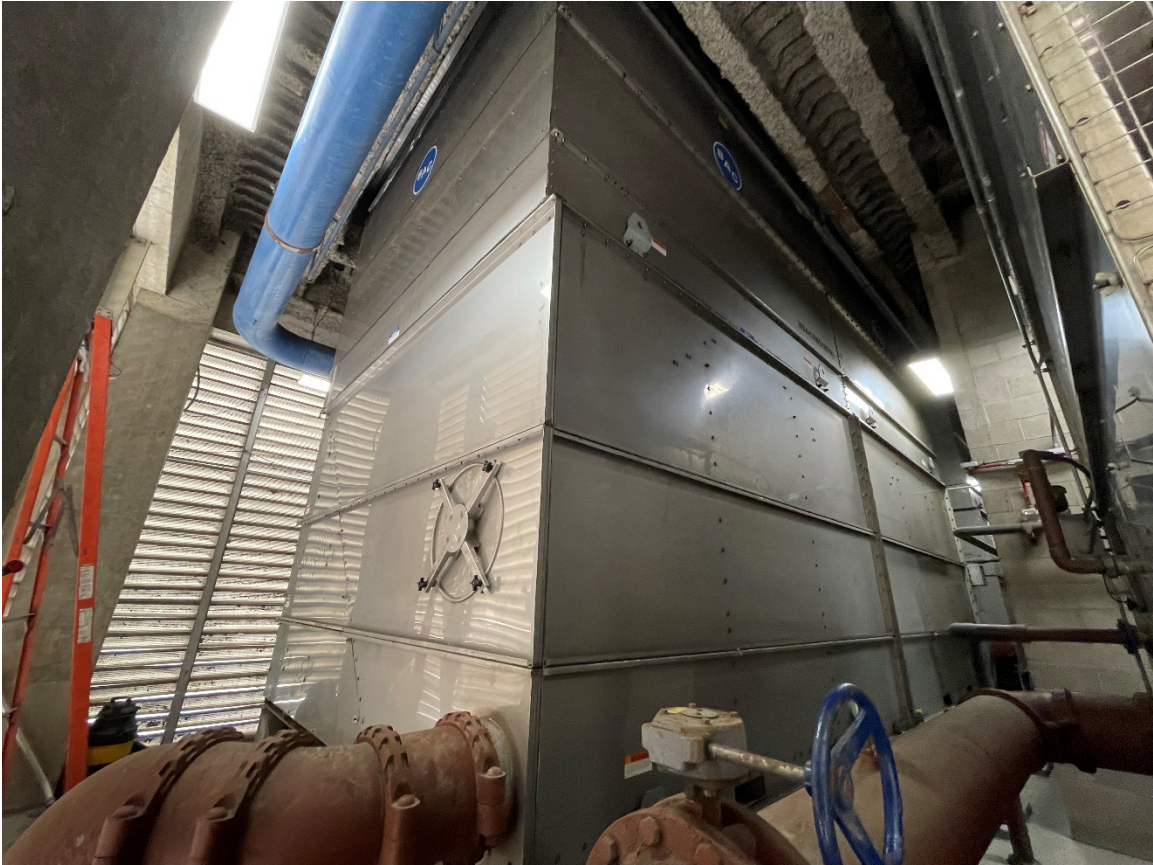
Cooling Tower #3 Lower Section (BAC VT1-800-Q #U164431105-02-01)
