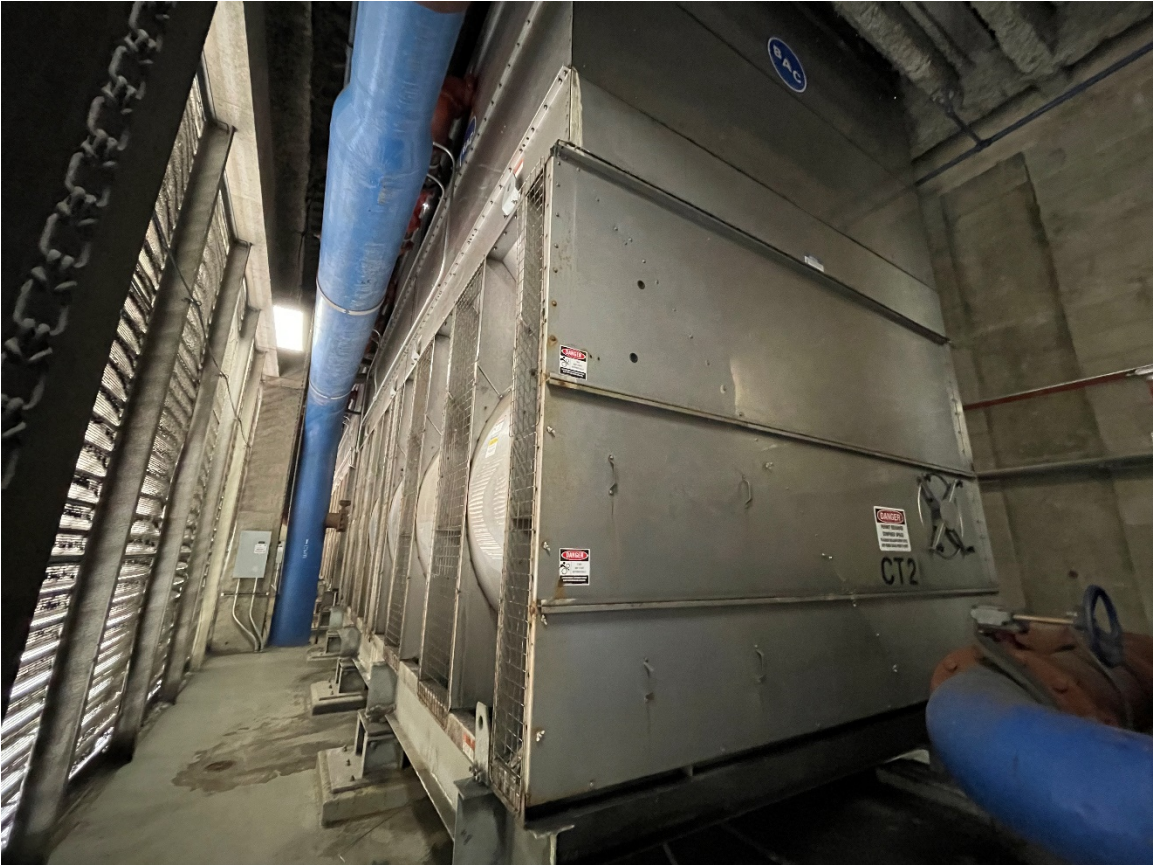
Cooling Tower #2 Lower Section (BAC VT1-800-Q #U164431105-03-01)
