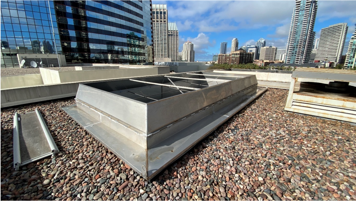
Cooling Tower #4 Top (BAC VT1-800-Q #U164431105-01-01)
