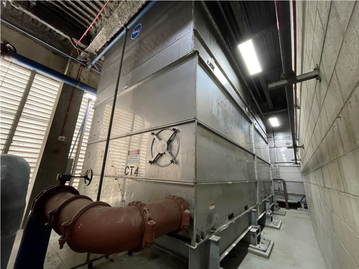
Cooling Tower #4 Lower Section (BAC VT1-800-Q #U164431105-01-01)
